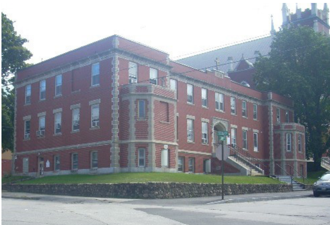
Expansion and renovations are already underway to serve more people on their recovery journey at St. Francis in Auburn.
