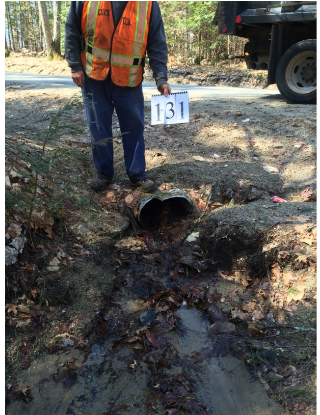
PHOTO: A culvert survey of town roads within the Kezar Lake watershed was completed in 2015. Each culvert was assessed and prioritized for replacement.
