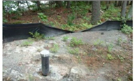
Silt Fence Not Trenched
