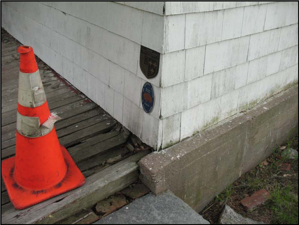
Photo EP6 – Concrete foundation fascia at deck and rotted deck.
