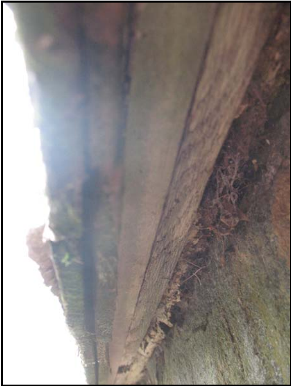
Photo EP4 - Base furring boards on old water table?
