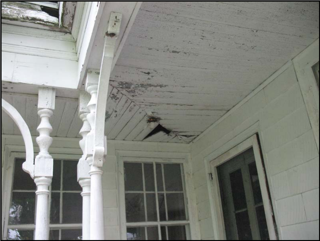
Photo EP8 – Deck ceiling rotting due to wall leaks above.
