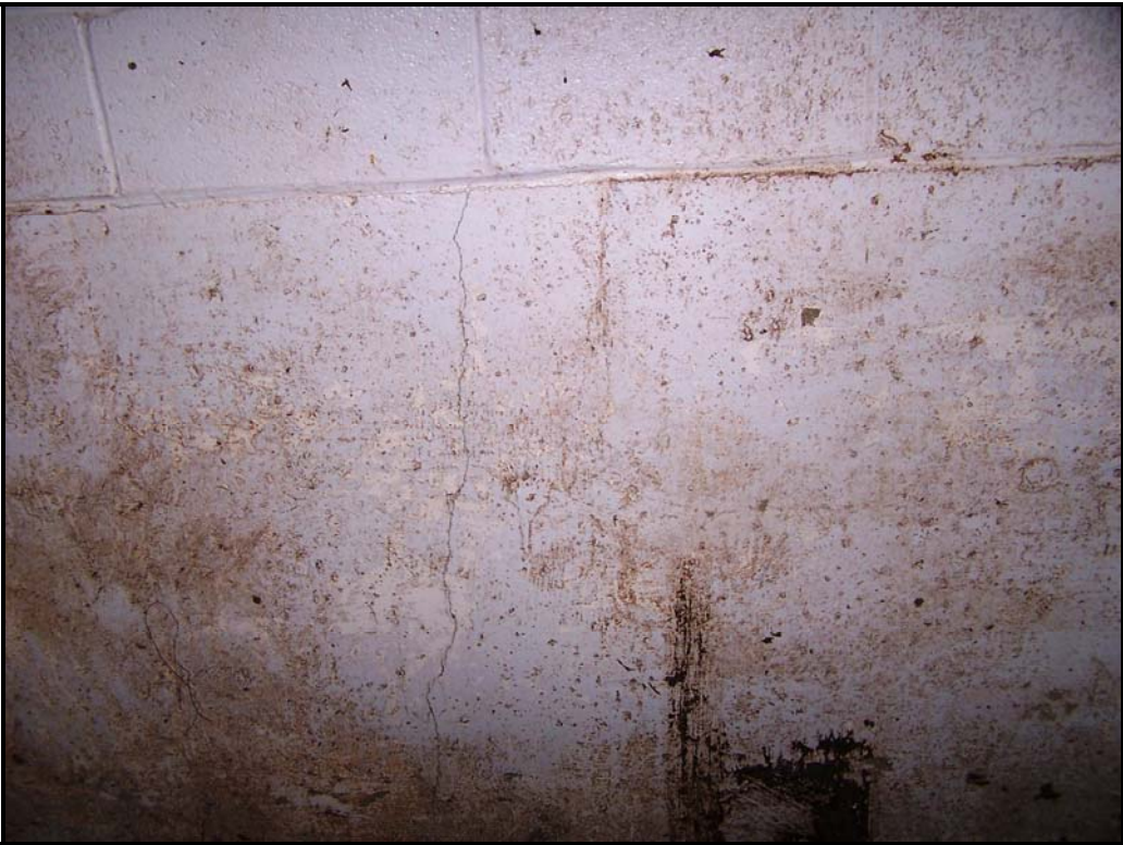
Photo BN18 – Minimal shrinkage crack in new milking barn foundation wall.
