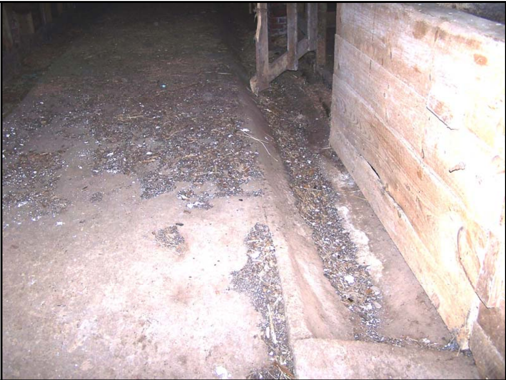
Photo BN14 – Raised basement slab in old milking room in basement of main barn.
