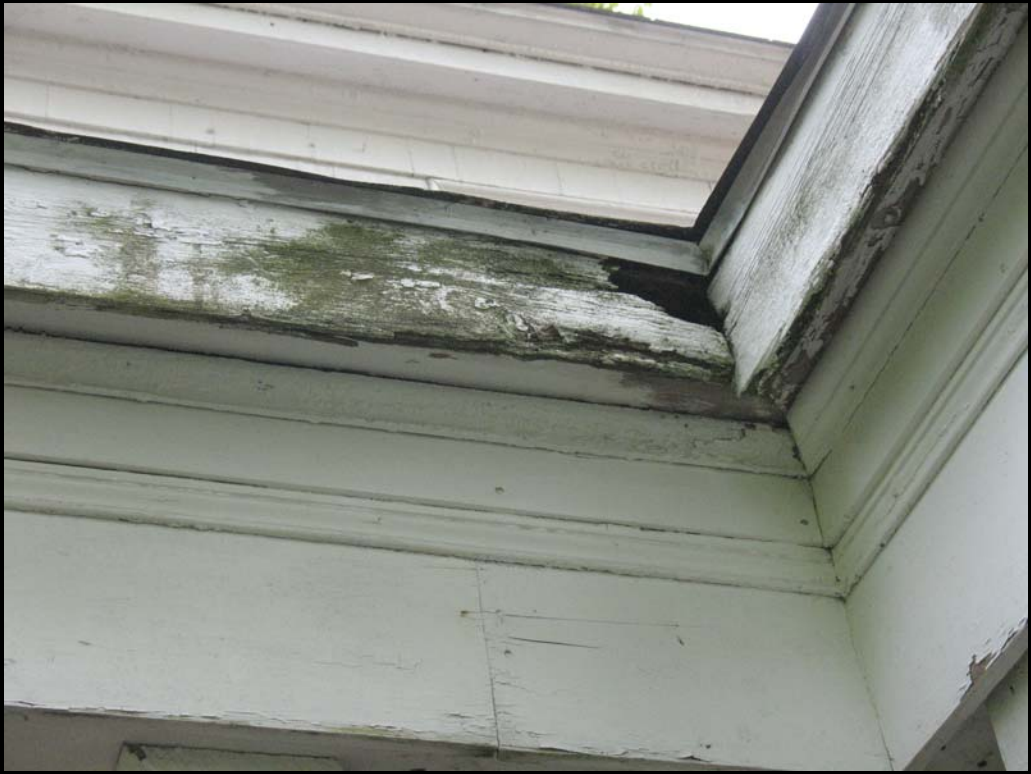
Photo EP9 - Deck roof fascia boards; rotted through.
