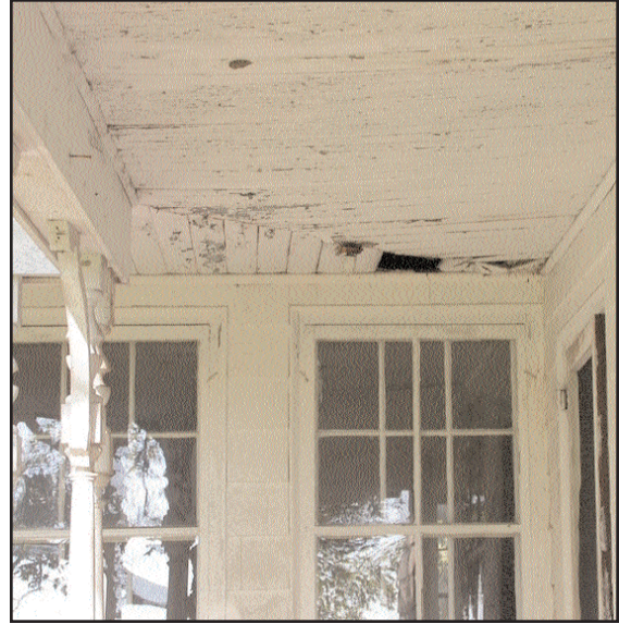
Figure 2: Deterioration of porch ceiling
