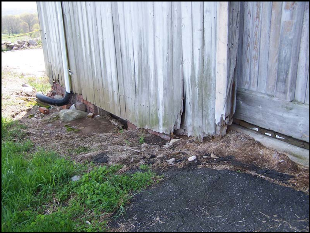
Photo BN21- 1908 barn foundation walls at corners needing repair.
