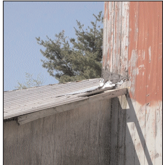
Deterioration of eave and sidewall flashing.
