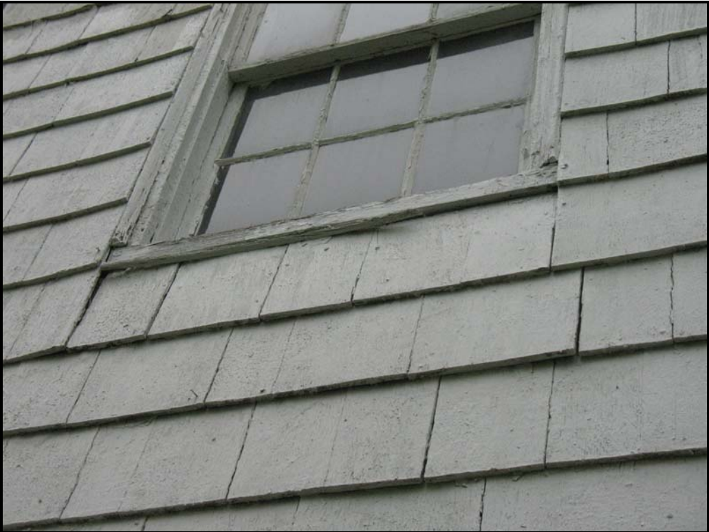
Photo EP10 – Window trim rotting due to extra shingle surface treatment.
