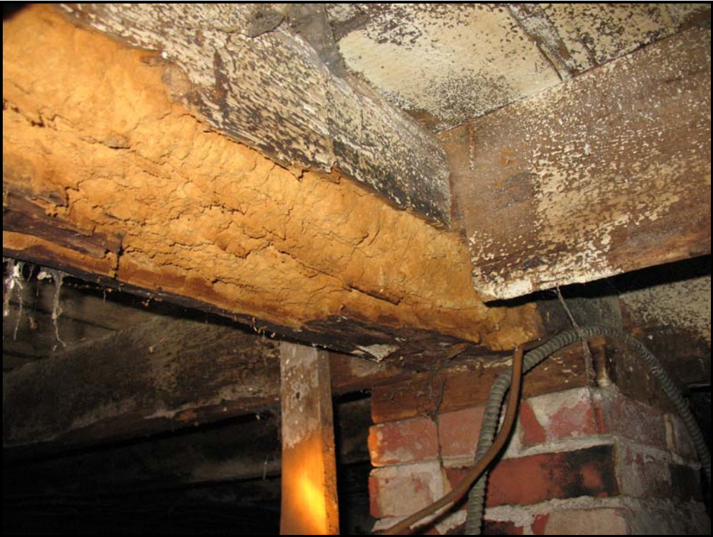
Photo B5 – Main House girder with heavy powder post beetle damage.
