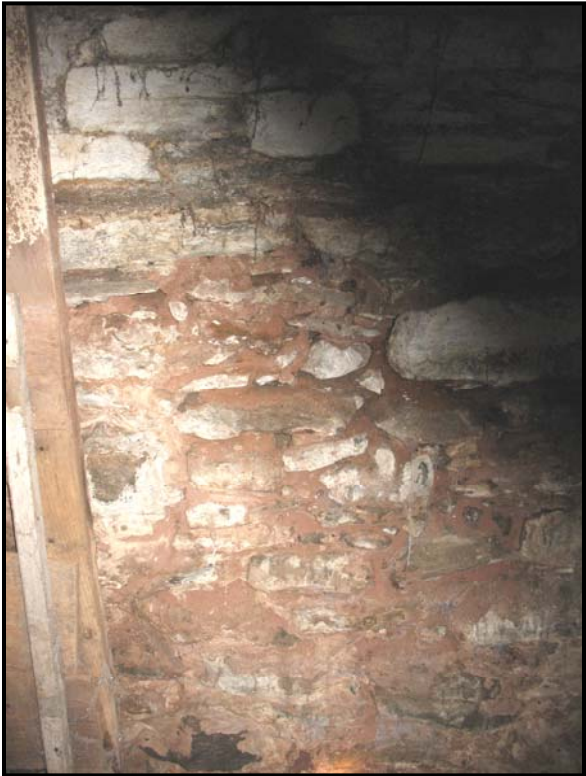
Photo B6 – Main House foundation wall with mud or lime mortar.
