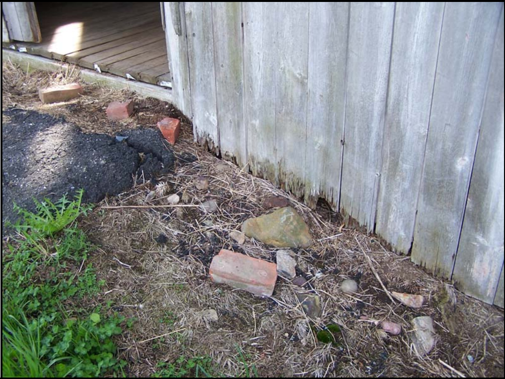
Photo BN22 – 1908 barn exterior wall with damage to adjacent raised soil grade.
