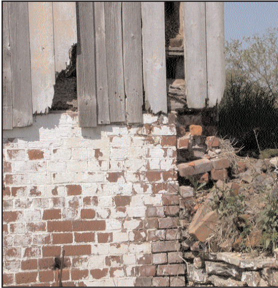
South east corner of 1908 barn. Note severe deterioration of masonry foundation and siding.
