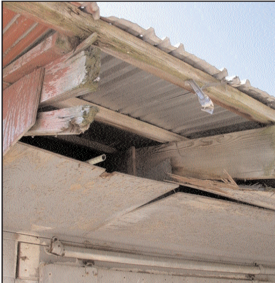
Deterioration of eave on north side of 1980 barn.
