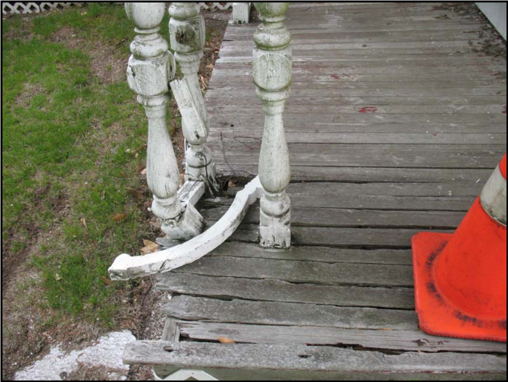
Photo EP7 – Deck corner rot with buckled porch columns.
