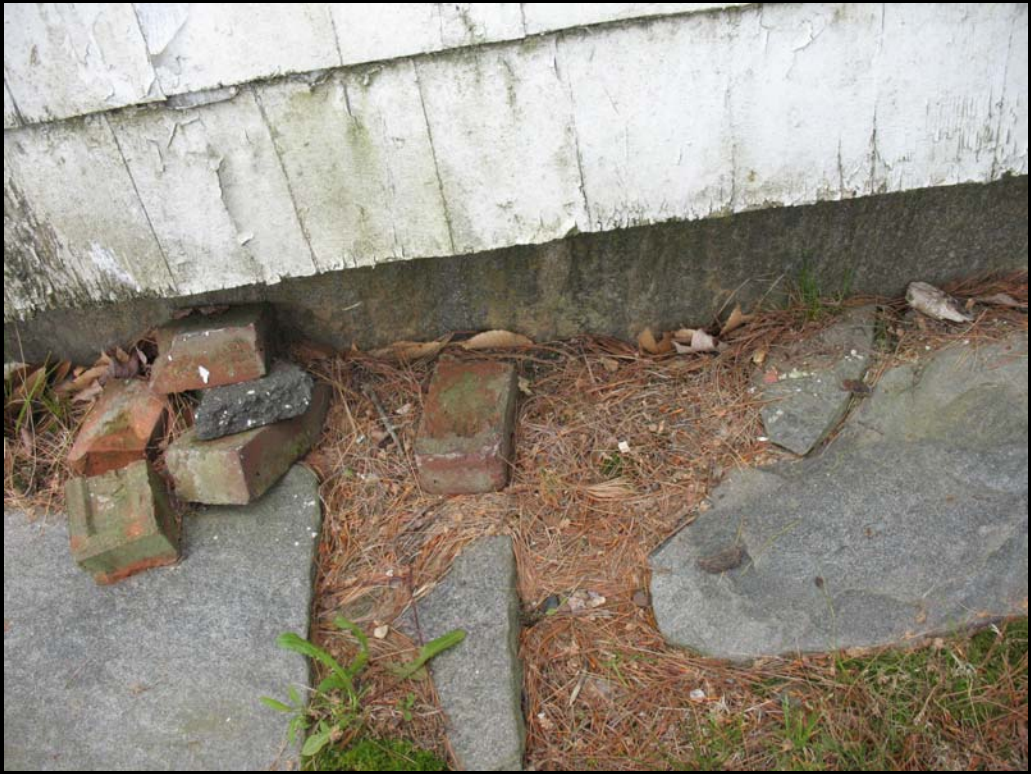
Photo EP3 – Projected shingles from recessed foundation wall.
