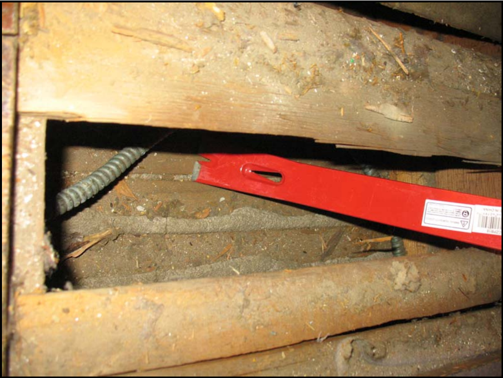
Photo P7 – Main house second floor indicating well keyed ceiling on wood lath below.
