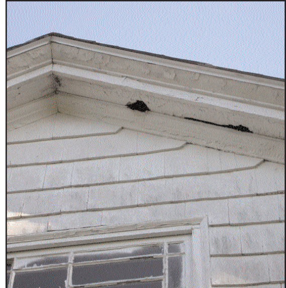
Figure 4: Eave at south wall of main house is badly deteriorated. The best time to rebuild an eave is when the roof is replaced.
