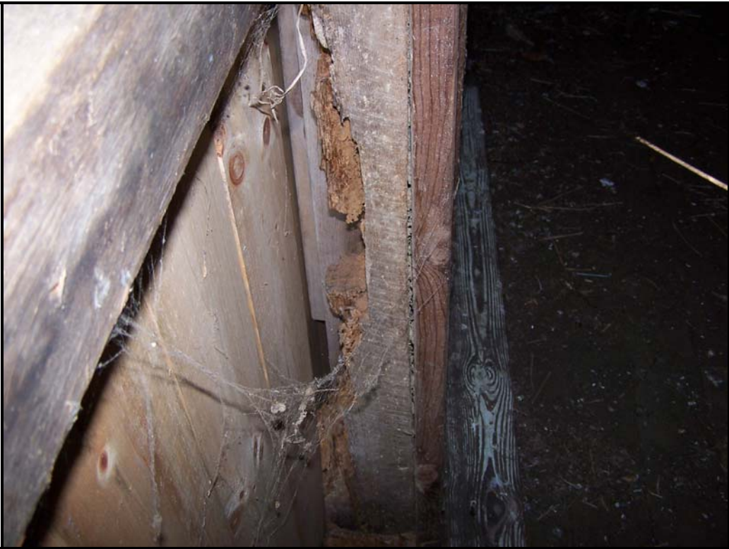
Photo BN2 – Main barn exterior post with powder post beetle damage.
