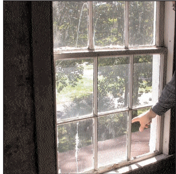
Replace broken or missing glazing (this window pane on east side of second floor fell out of frame and as found on porch roof).
