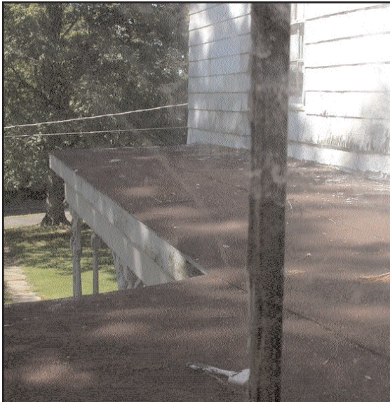
Figure 3: Porch roof past the end of its' useful life. Porch roof structure deteriorated. New sidewall flashing needs to extend under siding.
