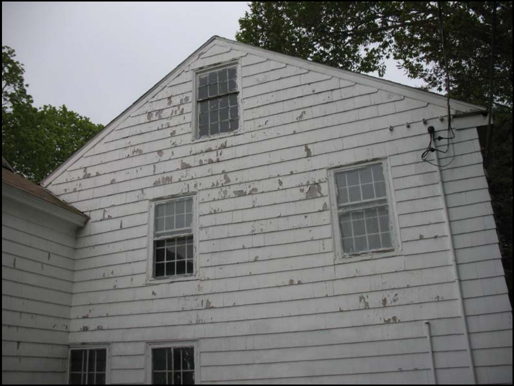
Photo EP11 – Paint peeling due to trapped moisture in shingles.
