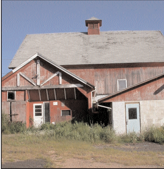
Figure 1: Deterioration of barn roof.
