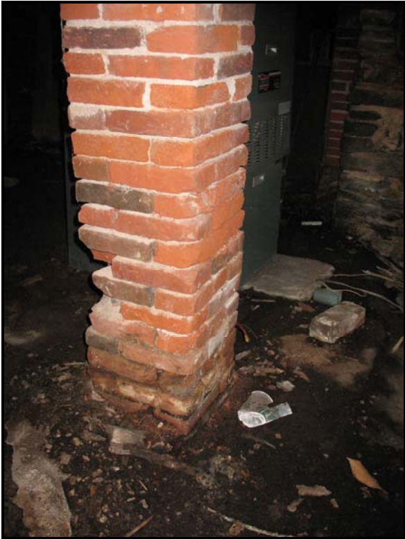
Photo B3 – Heavy brick pier damage at Main House.
