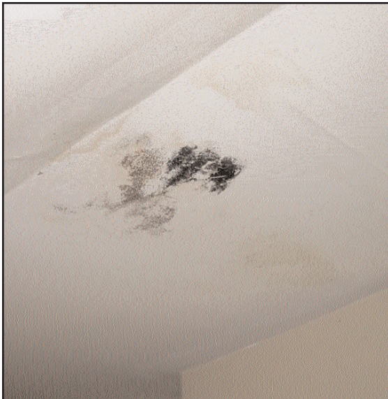
Mold on second floor ceiling of kitchen ell. In an unheated building mould will grow on the paper cover of gypsum wall-board.
