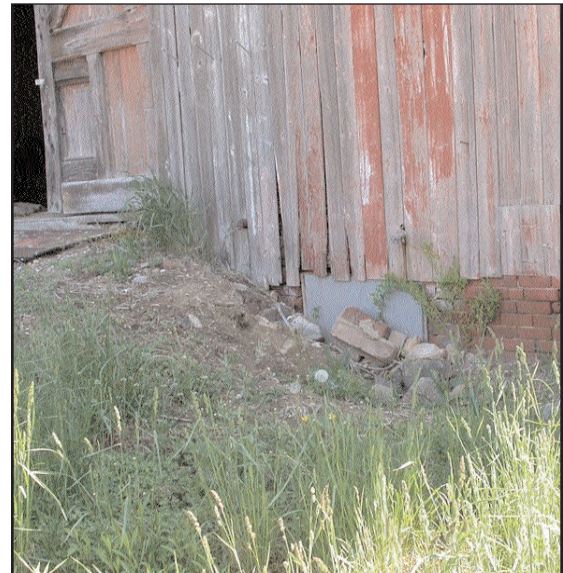
Deterioration of siding adjacent to grade west side.
