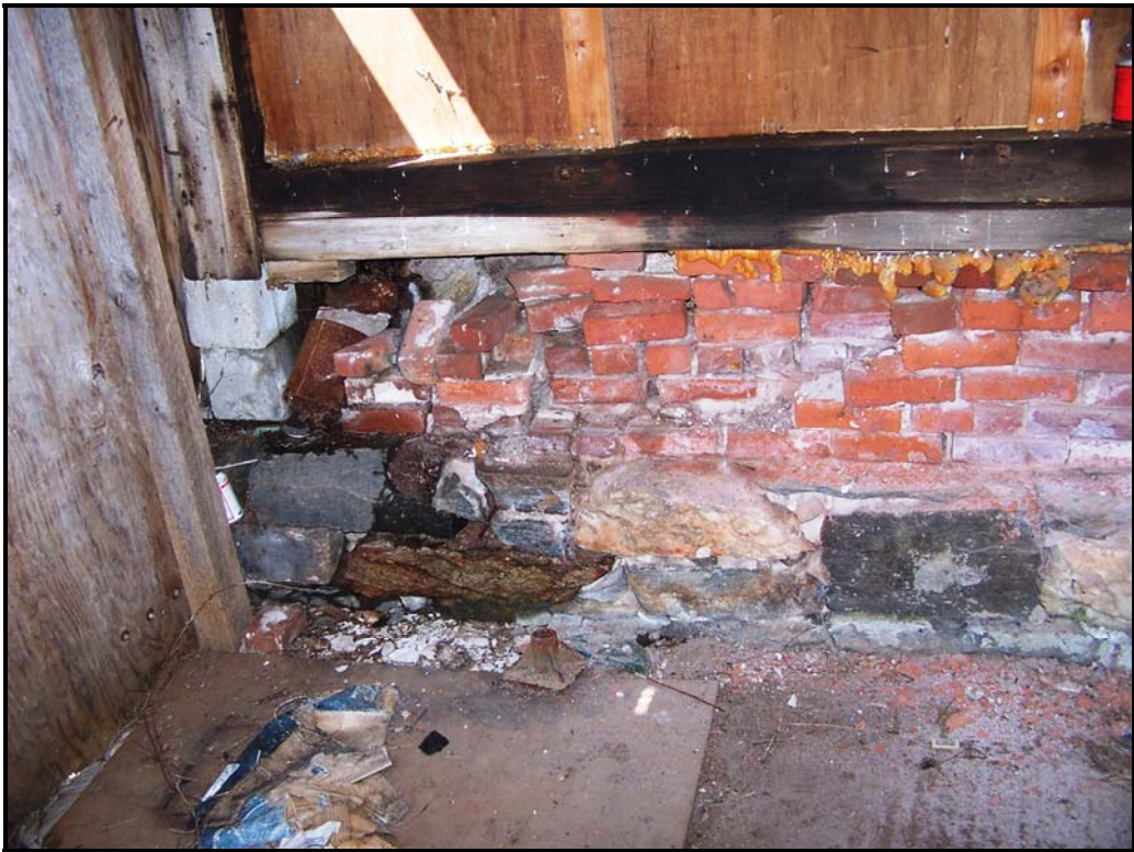
Photo BN11- Collapsing front foundation corner on the south shed building.
