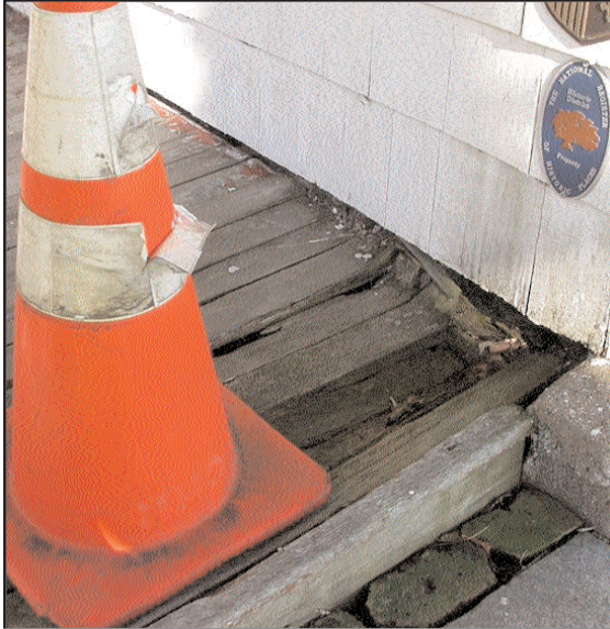
Figure 1: Deterioration of porch structure and finish.
