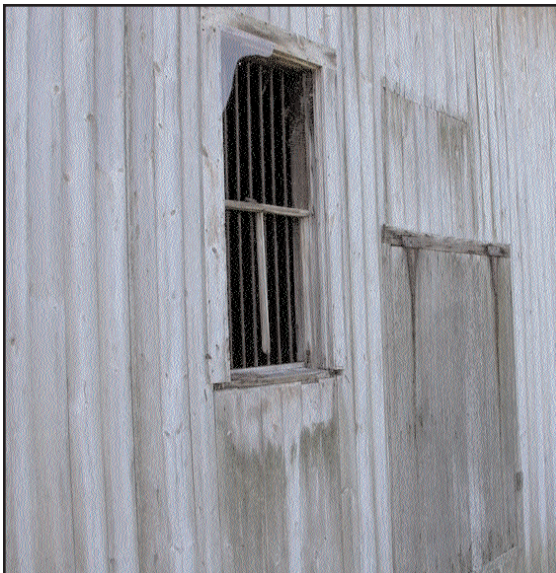
Window opening with deteriorated enclosure.
