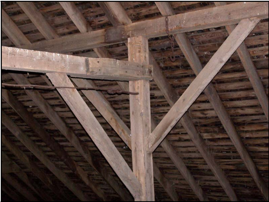
Photo BN5 – Main barn cross frame showing scabbed on repair pieces at timber end connections.
