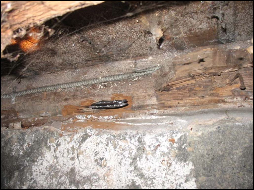
Photo B1 – North side Main House sill rotting.
