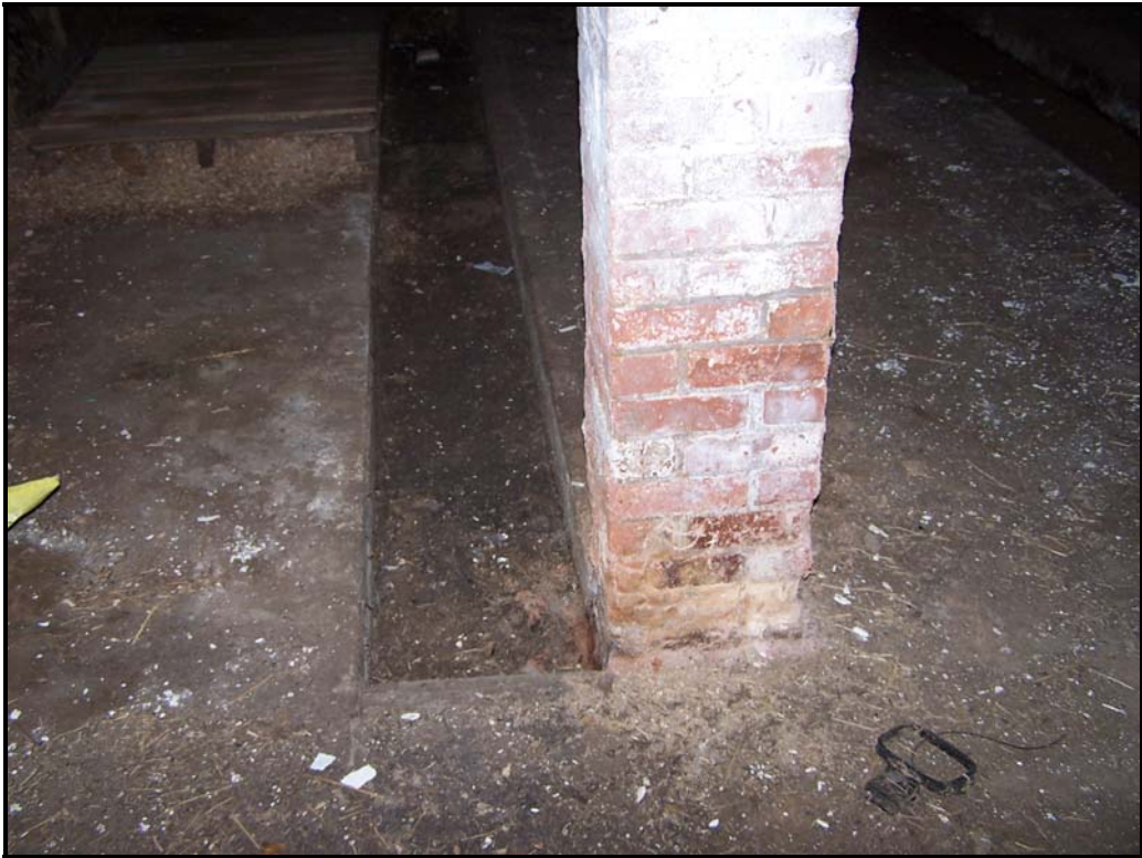
Photo BN12 – Deteriorating base of main barn basement brick pier.
