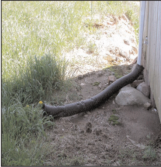
Rainwater leader terminates "uphill". Rainwater leaders to be connected to fence drain and connected to drywell.
