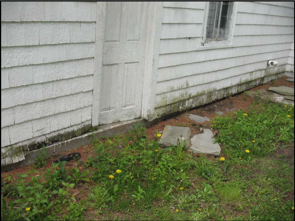
Photo EP12 – Base course shingle rotting due to roof runoff splash zone.
