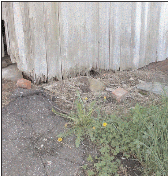
Deterioration of siding adjacent to ramp area north side. Grade/ramp access to be reworked to remove grade from wood cladding / framing.
