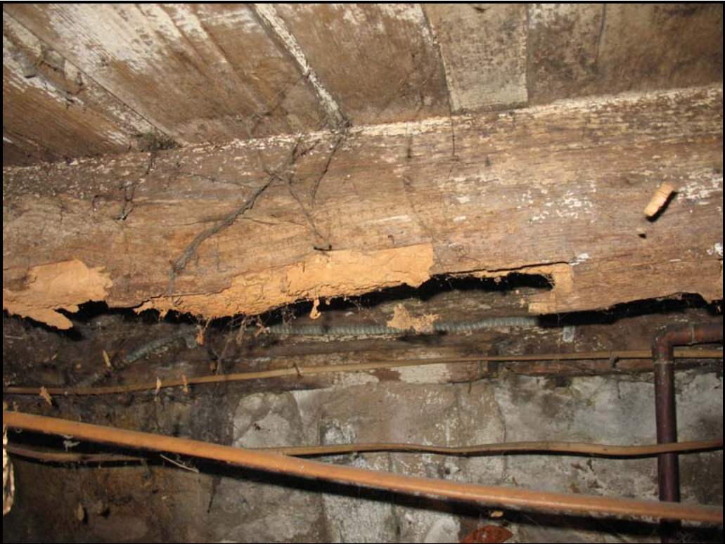
Photo B2 – Main House first floor joist with severe powder post beetle damage.
