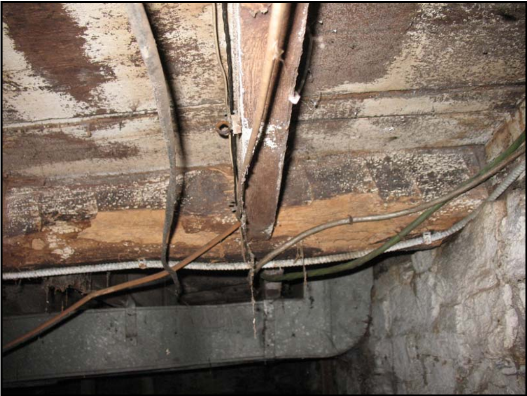
Photo B4 – Main House girder damage at front (south) wall.
