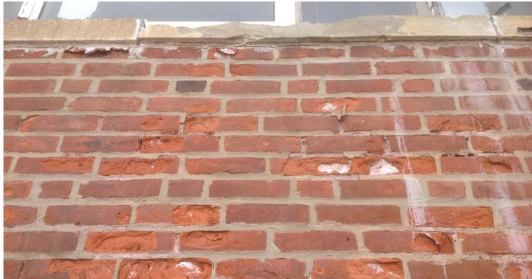
Brick Spalling and Concrete Sill Deterioration
