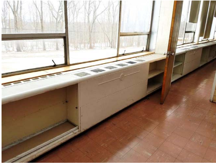
Typical Classroom Unit Ventilator
