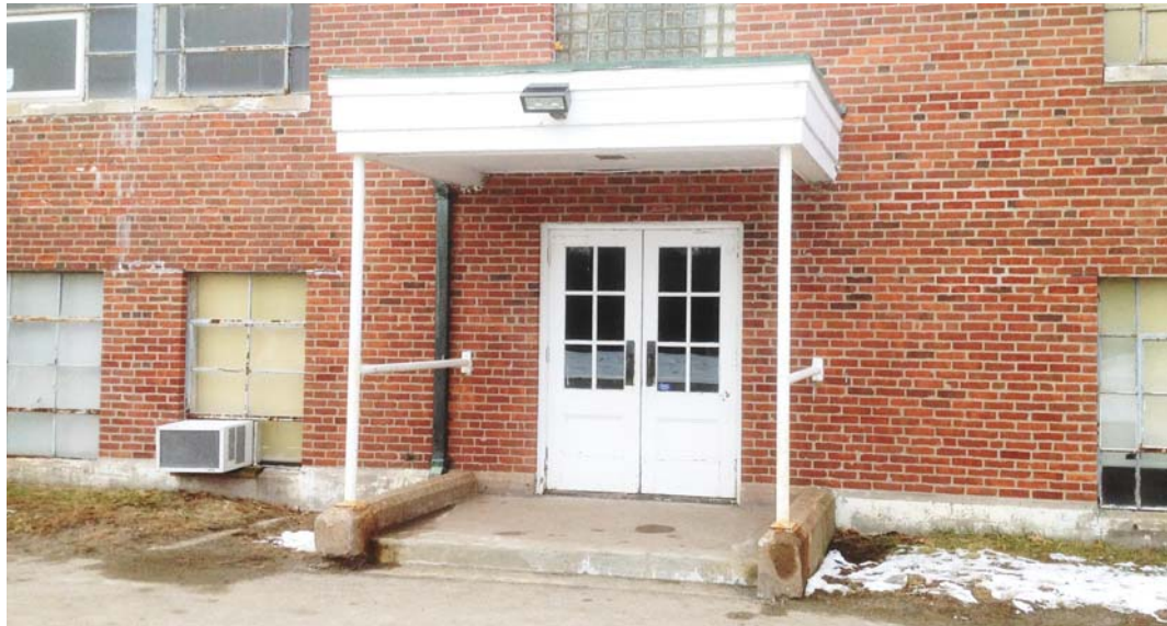
Stair Egress Canopy at East Side (Note - Single Riser is Not Permitted by Code)
