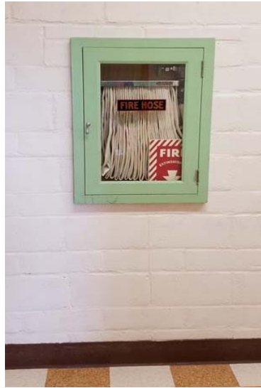
Typical Hose Valve Cabinet
