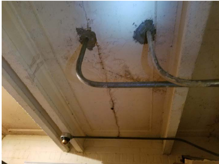
Slab Crack on Underside of Slab
