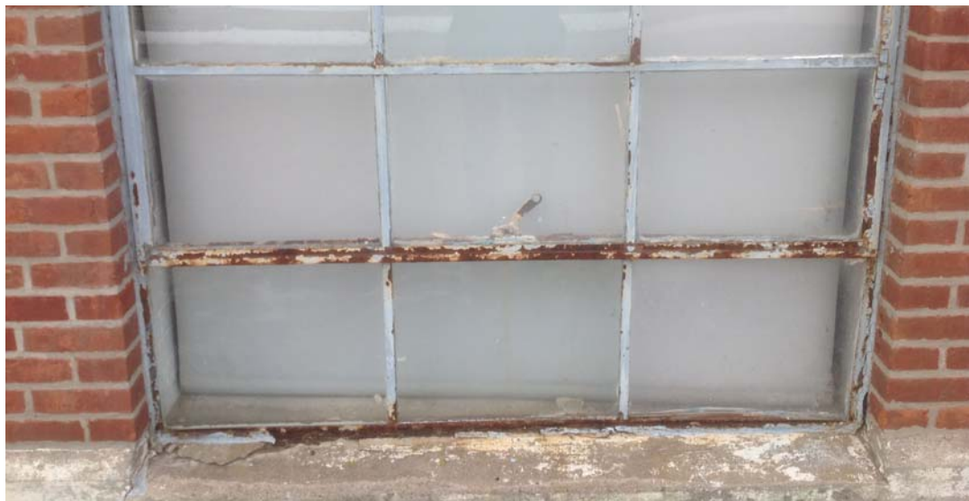
Close-Up of Typical Steel Window Condition
