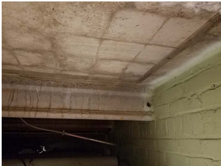
Mesh Pattern on Underside of Slab
