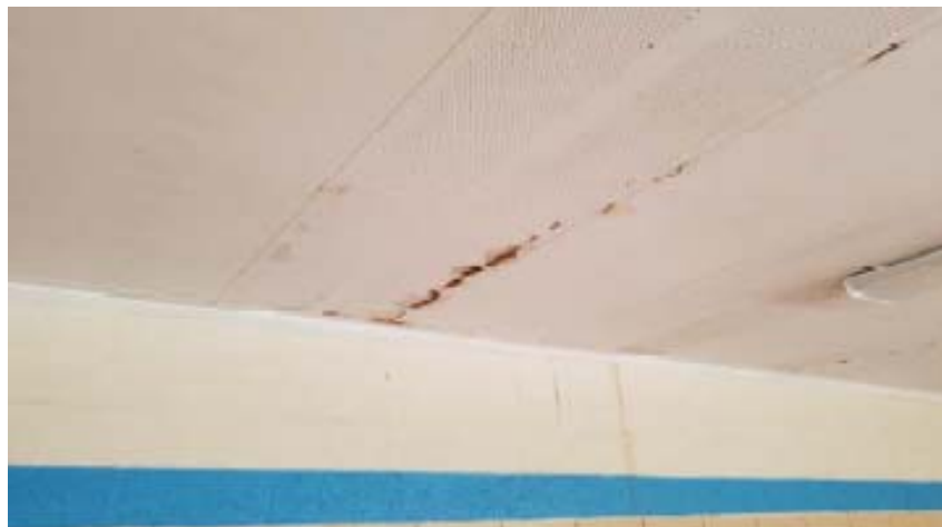
Corrosion of Metal Decking
