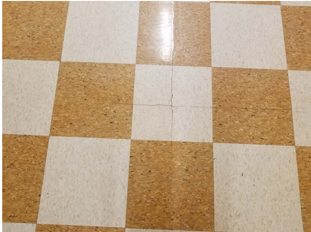
Cracks in Main Level Flooring
