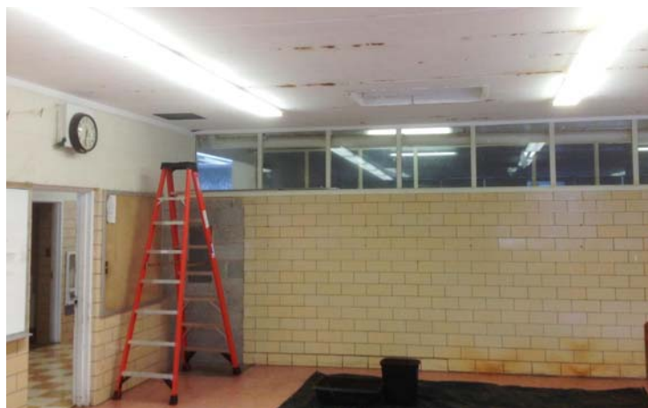
Upper Level Classroom Showing Water Damage
