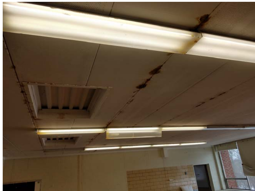
Corosion of Metal Decking
