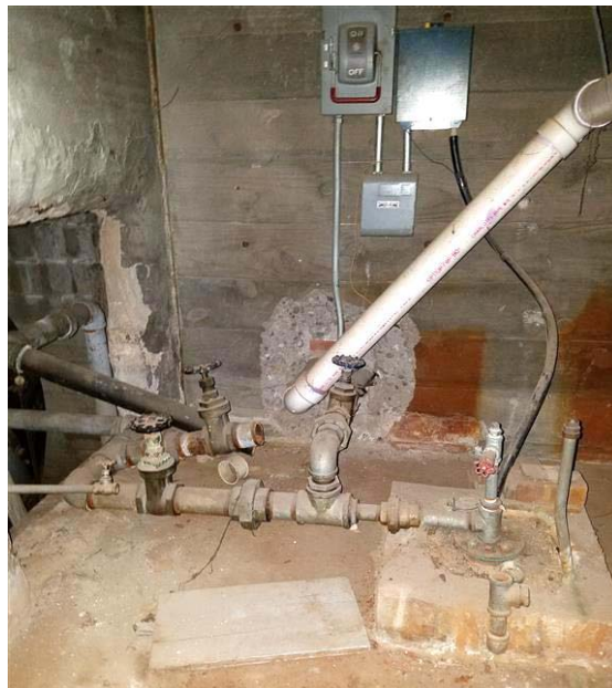
Incoming Water Service
