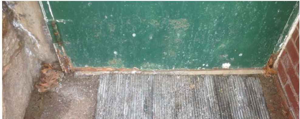
North Wing Lower Level East Door - Rusted Door and Frame Bottom
