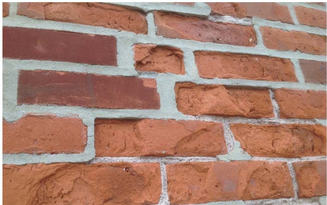
Close Up of Brick Spalling
