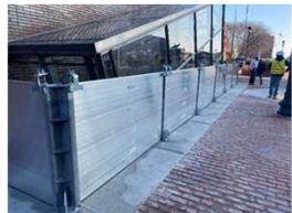
Stop Logs, Aquarium Station, Boston, MA
