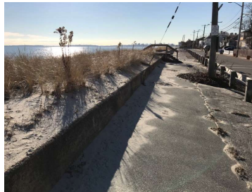
Sand overtopping seawall
