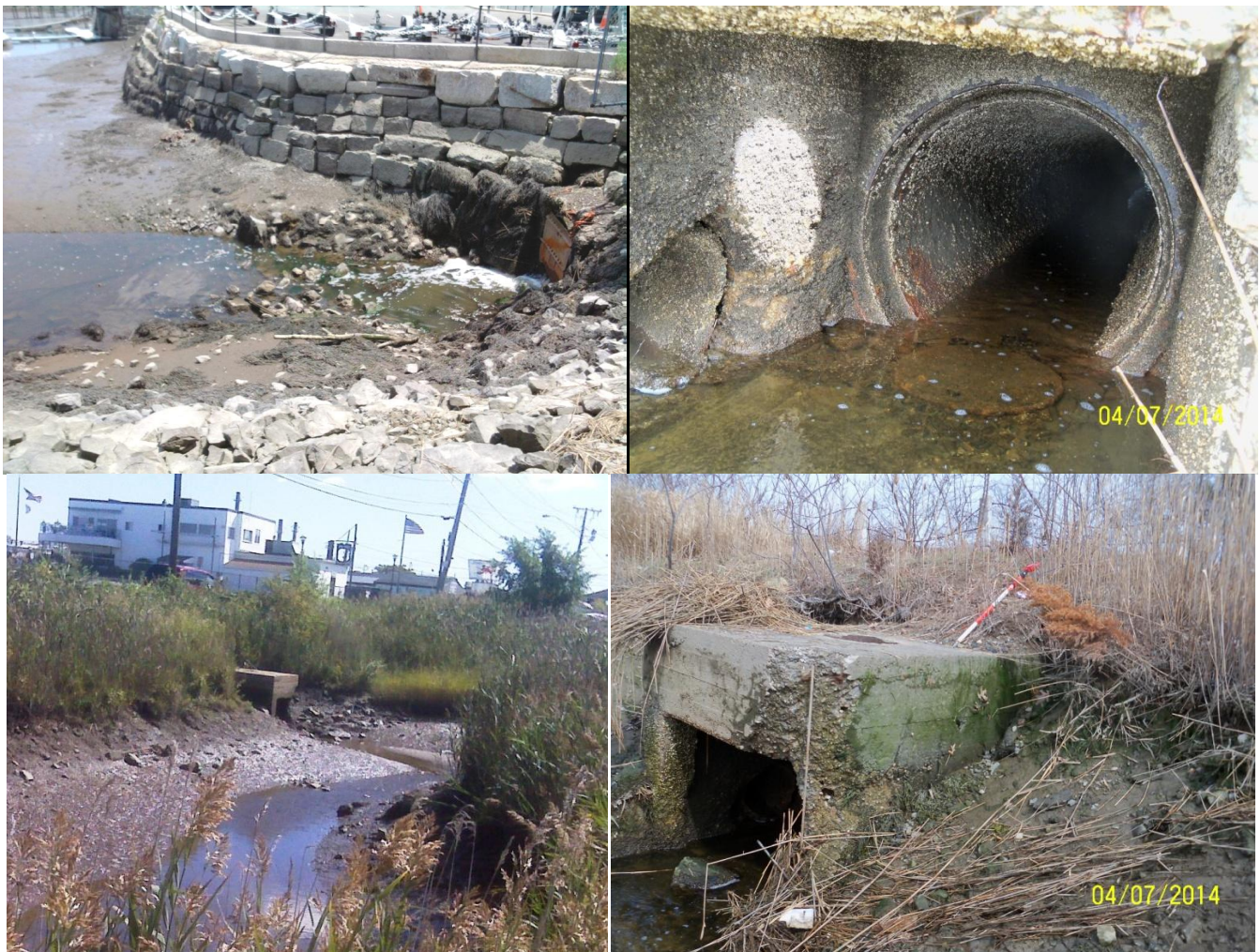
Fig. 2.19: Ballard Street Culvert (“BA-1”) Upper Left: Flap Gate on Downstream End of Ballard Street Culvert Upper Right: View of 48-In. pipe in Upstream Manhole Lower Left and Right: Rectangular Manhole at Upstream End of Ballard Street Culvert
