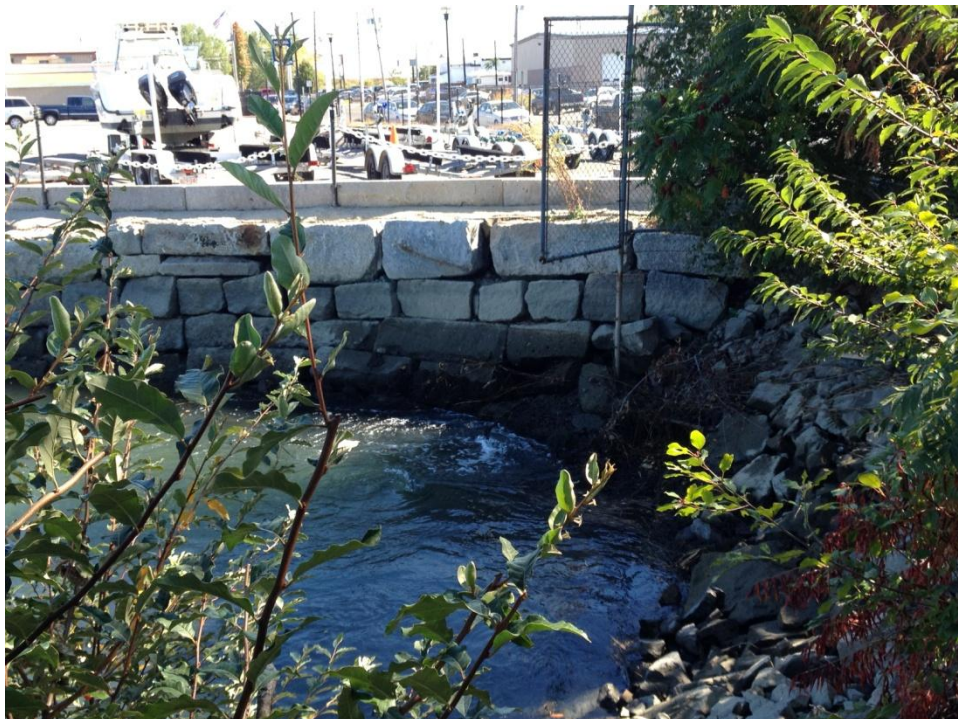
Fig. 2.28 Ballard Street Culvert (“BA-1”) flowing full with no headroom at mid-tide.
