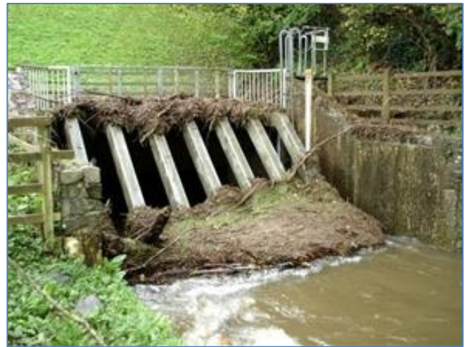
Fig. 3.01 Blocked culvert grate (“trash rack”) with wide bar spacing (photo credit: environment-agency.gov.uk).
