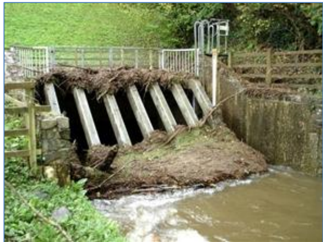
Fig. 3 Blocked culvert grate (“trash rack”) with wide bar spacing (photo credit: environment-agency.gov.uk).
