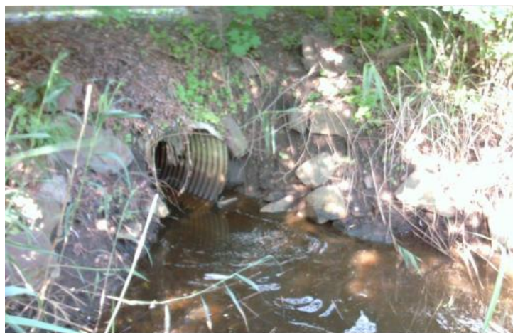
Fig. 2.13 Downstream end of Eastern Avenue Ditch Connecting Culvert “E-5” (Photo by Woods Hole Group, Inc., Appendix 1)
