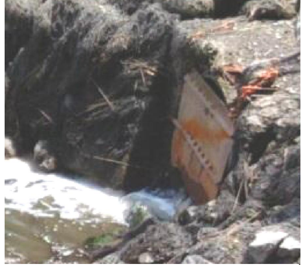
Fig. 4.10 Enlarged View of Improvised Tide Gate on North End of Ballard Street Culvert
