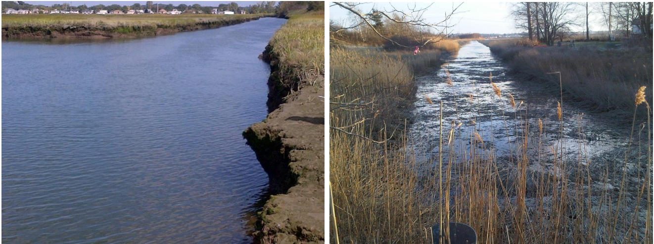
Fig. 2.24 Pines River Channel, along the west side of the I-95 embankment Left: Looking north from a point south of the tide gauge location. Right: Looking south from Bristow Street
