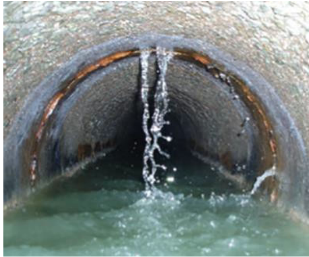
Infiltration into a sanitary sewer
