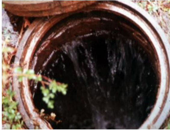
Inflow into a manhole
