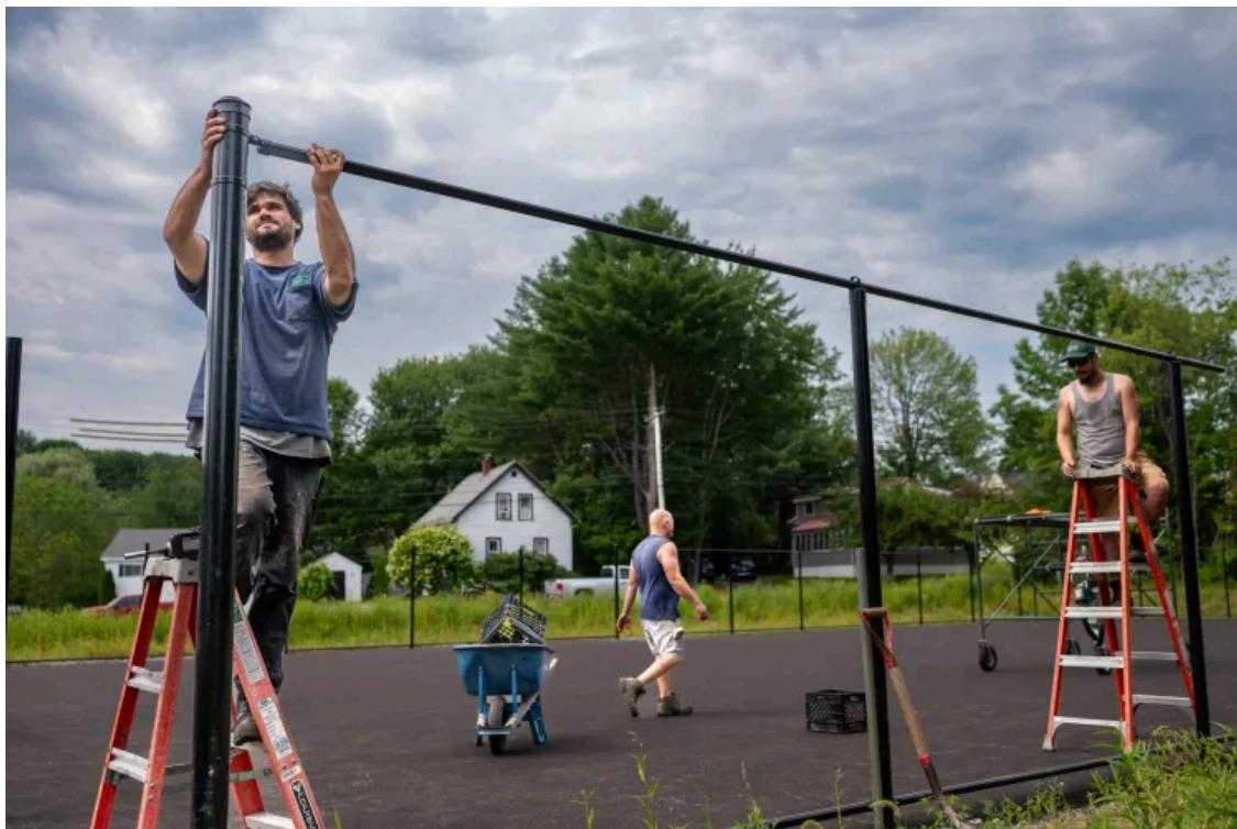
Matt Kasabian, left, of Main Line Fence, connects the top of a fence section Monday at the new pickle ball courts being constructed on North Temple Street in Lewiston. Andree Kehn/Sun Journal
