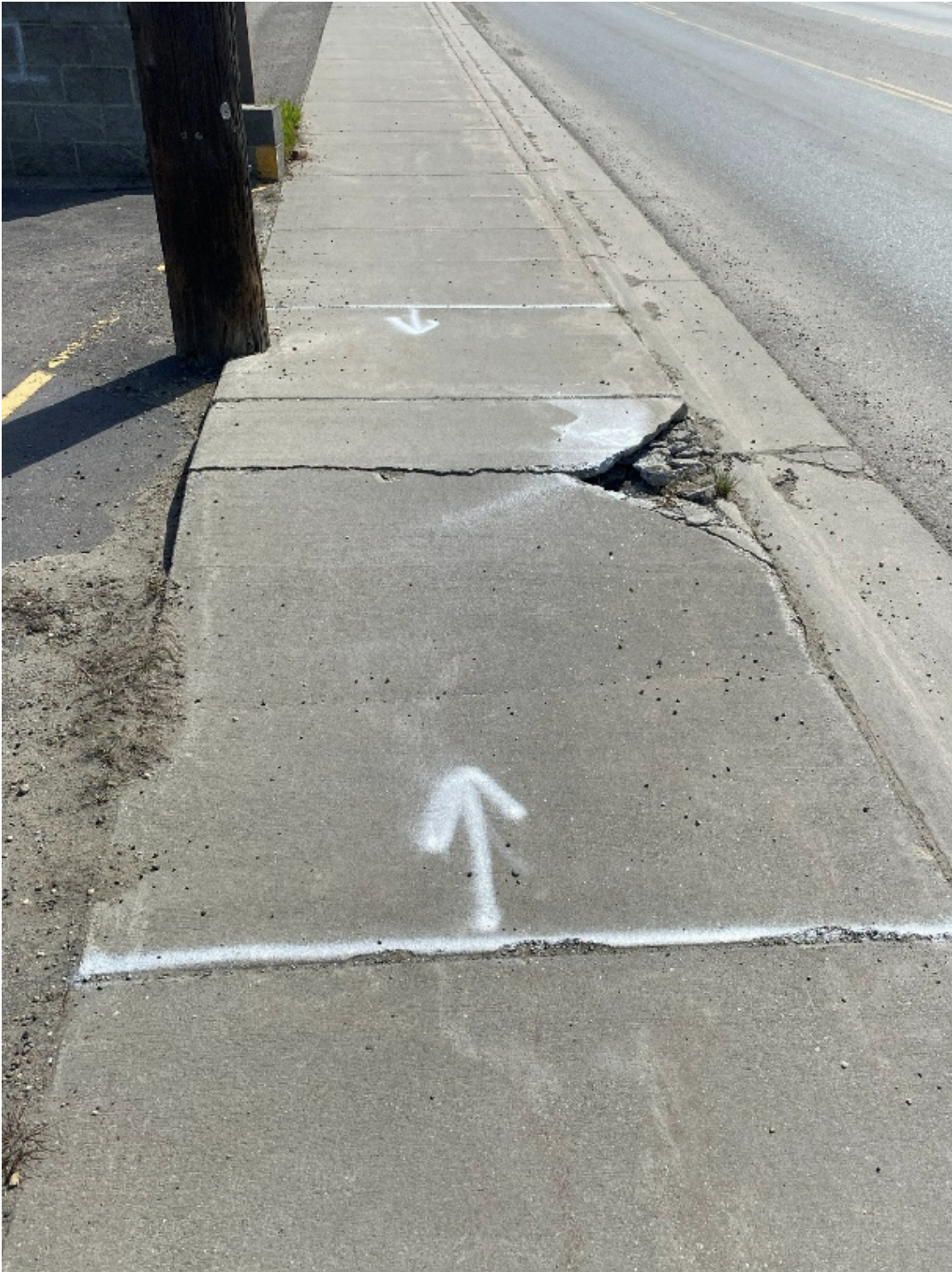
Figure 4. Street Sounds, South Cushman Street; DUCT BANK WARNING!
