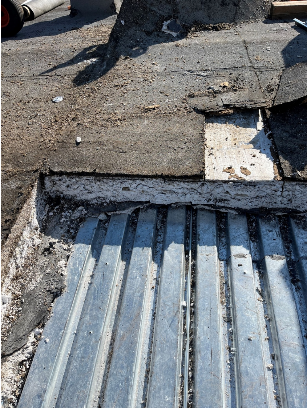
METAL PAN BENEATH SECTION A ROOF DURING DEMO FOR GENERAL REFERENCE. NOTE: EXISTING CONDITIONS OF SECTION B ROOF MAY DIFFER.
